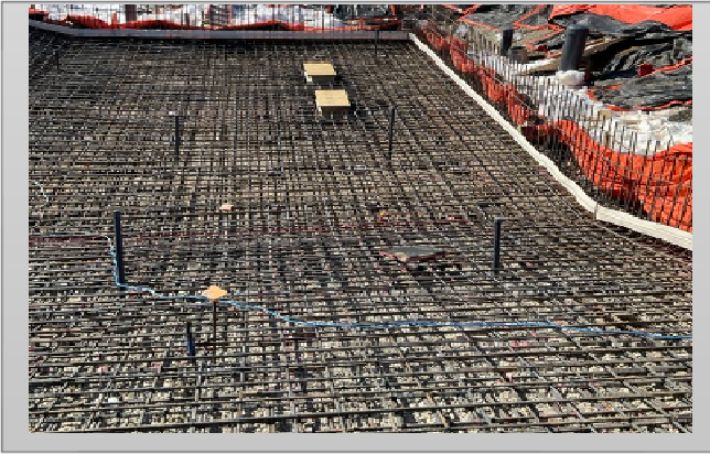
Rebar fully installed in lap pool floor, looking from shallow end down to deep end
