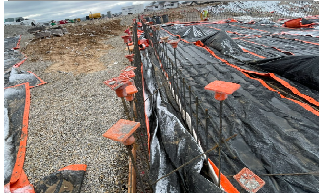
Lap pool floor covered for the weekend and wall rebar install beginning
