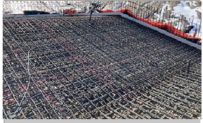
Rebar installed in lap pool floor, looking @ slope from shallow to deep end
