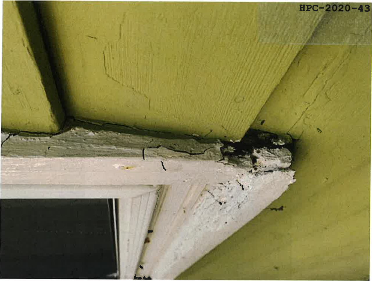
Bedroom window - not original - first floor · severe rot · inefficient
