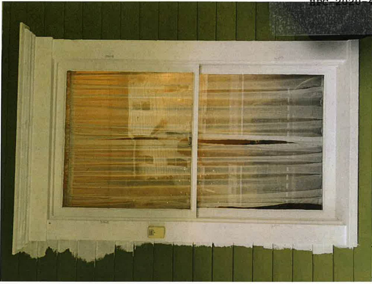
(North) First floor dining room - - giant single pane window - painted shut long ago - inefficient.
