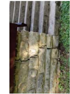
FIG. 2.6: WARMING HOUSE DETERIORATION
